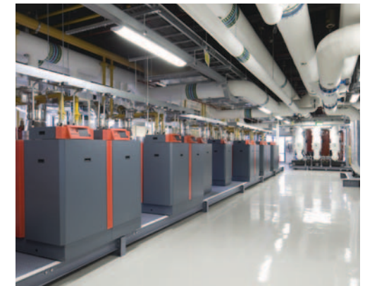
One Canada Square – new boiler room
